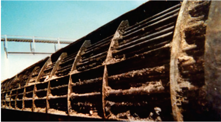
FIGURE 2: INTERSTAGE COOLER AFTER 5 YEARS ON LINE (RUN 1)
